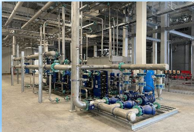
Water Cooling system
